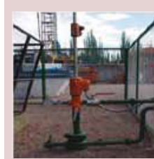
Stuffing Box, Production Tee, BOP Valve and APA
